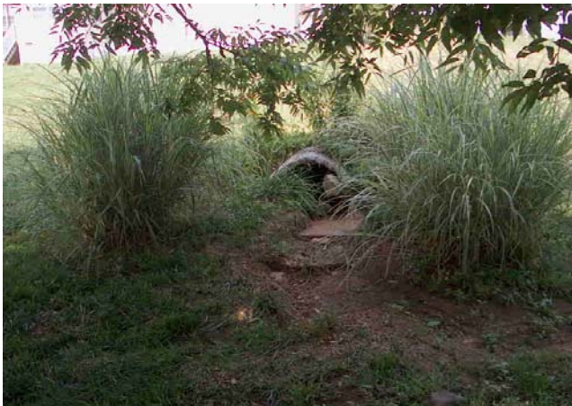
Poorly maintained and damaged inlets can cause flooding and property damage.
