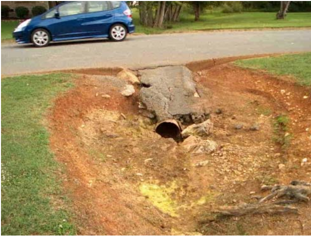
Eroded swales are unsightly, contribute to sediment loading to streams and can eat away at usable property for a homeowner.
